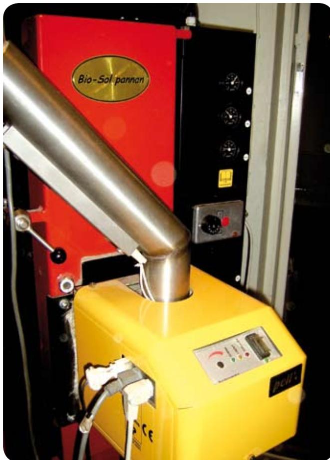
Biofuel pellets boiler and solar heat accumulator in the basement of the house (Photographer Christer Bjork)
