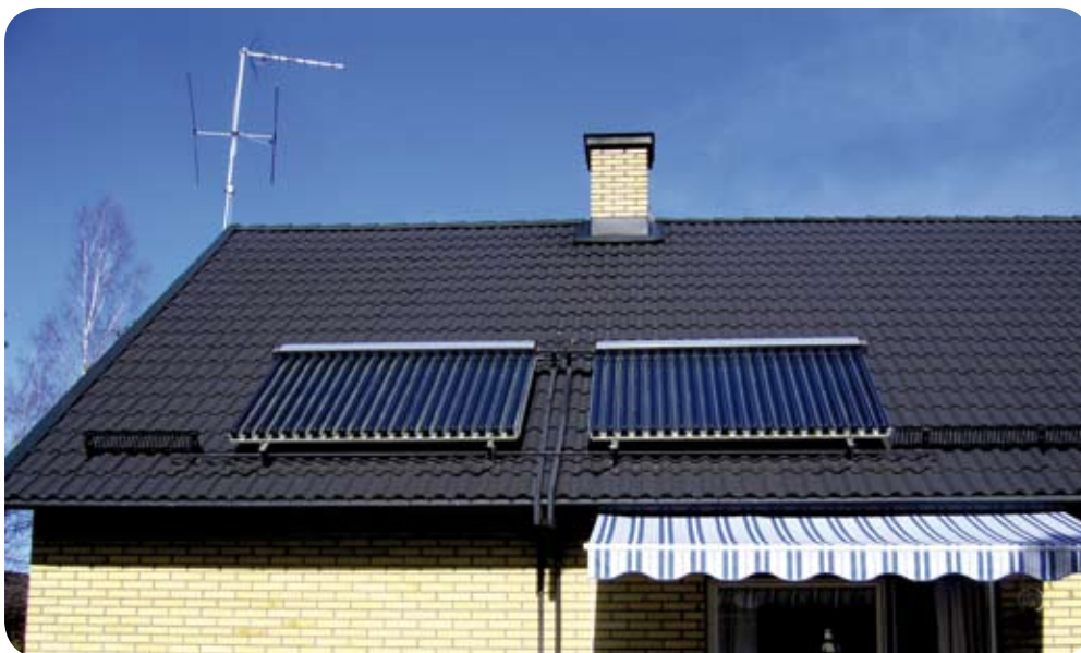
Solar collectors installed on the roof (Photographer Christer Bjork)
