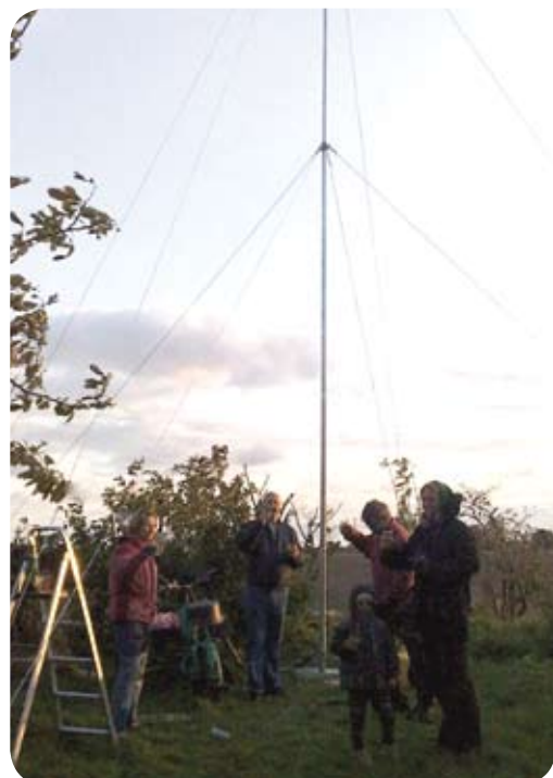
House owner's friends and the seller of the equipment helped to install the wind plant (Photographer Holger Wendt)
