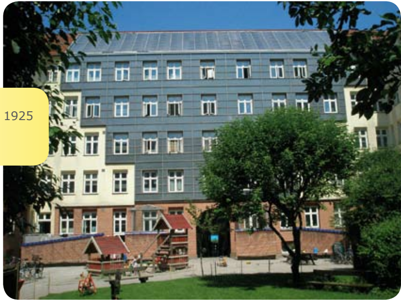
Solar collectors were installed on the buildings' front-wall (Photographer author Soren Dyck-Madsen)
